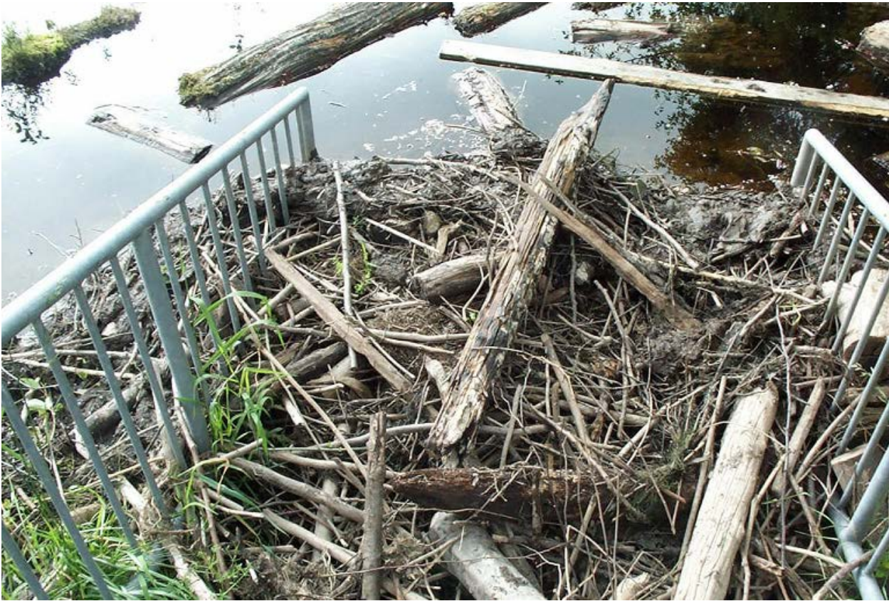
Beaver dam at the trash rack showing woody debris and mud
