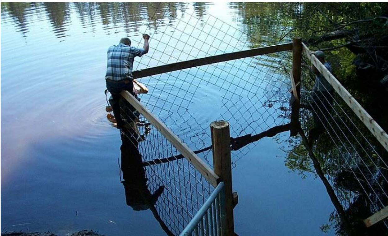
Last section being lowered into place. Note the hole cut out for the pipe to extend through.
