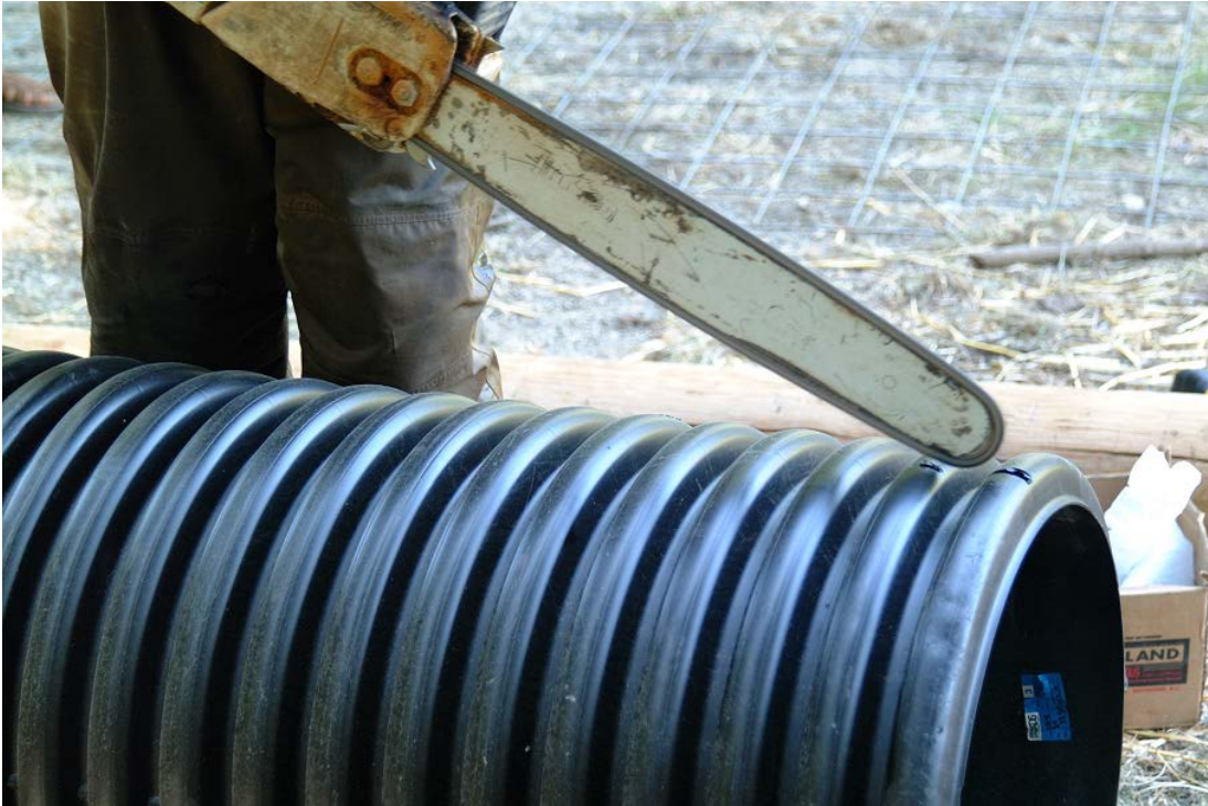
Cutting holes in the pipe to allow trapped air to escape and the pipe to sink.
